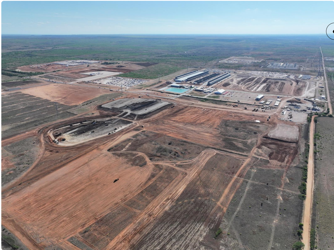
Galaxy’s Helios Data Center campus, April 2026.
